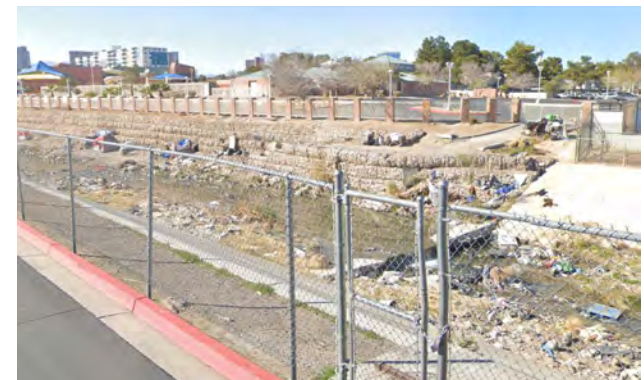
Lack of maintenance
