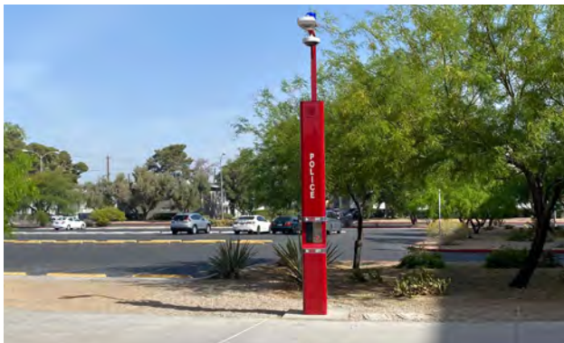
Emergency light box on UNLV campus
